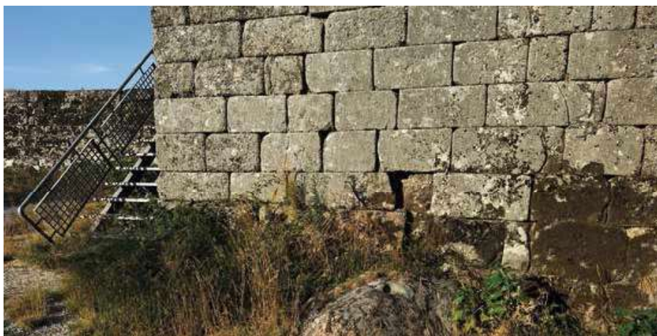
Ashlars from the tower's base and the adjacent wall. Detail.
